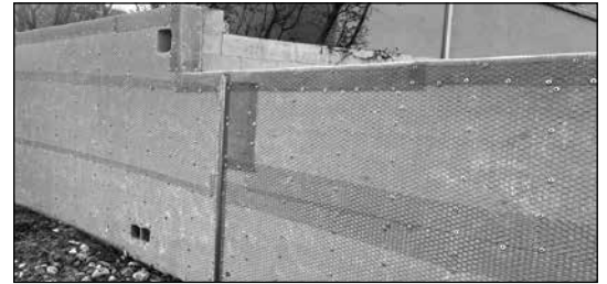
This portion of the Piñon Point wall along Spain is currently undergoing repair using chicken wire and metal mesh after the previous stucco failed to adhere.
